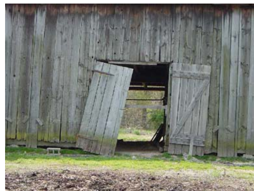
Doors in bad repair are left open until fixed.
