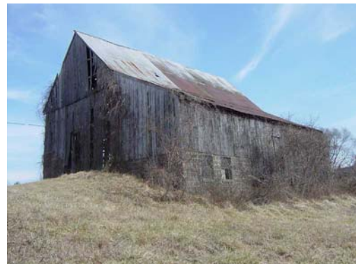
Vegetation is damaging this barn.
